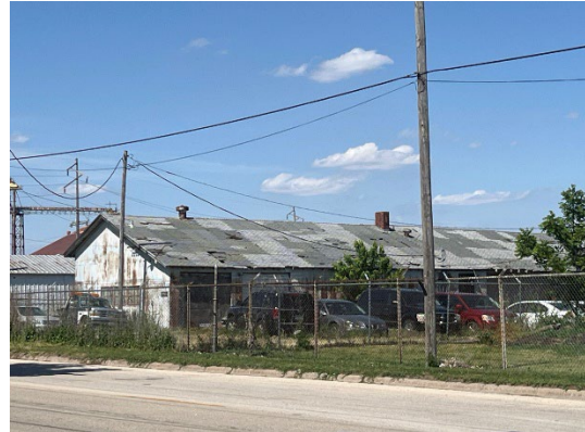
Weathered and deteriorated reroofing material deteriorated exterior walls.
