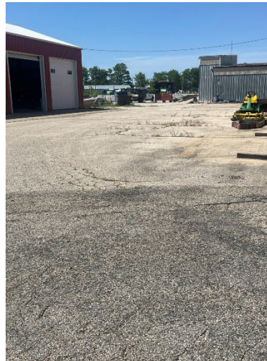
Deteriorated gravel lot which has resulted in vegetation growing in the cracks.
