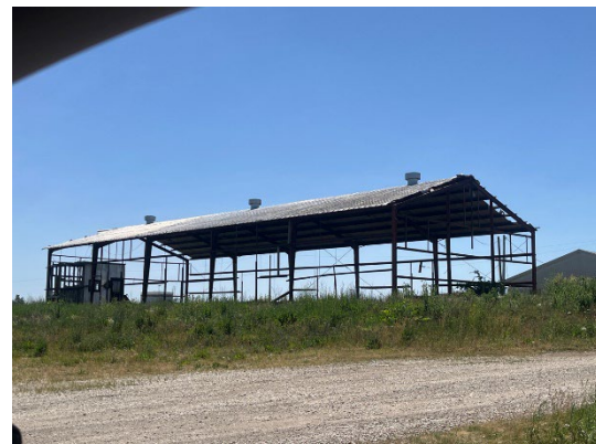
Exposed structural framing, roof failure.
