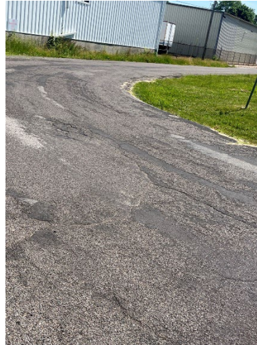
Deteriorated street pavement.
