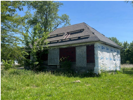
Vacant residential structure, boarded windows, overgrown vegetation.
