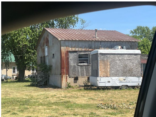
Corrosion and rusting of exterior metal panels, aging roofing materials.
