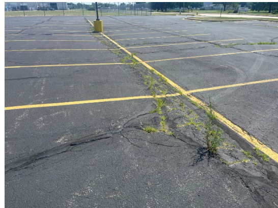
Deteriorated parking lot pavement which has resulted in vegetation growing in the cracks.
