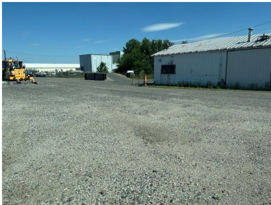
Deteriorated gravel lot.
