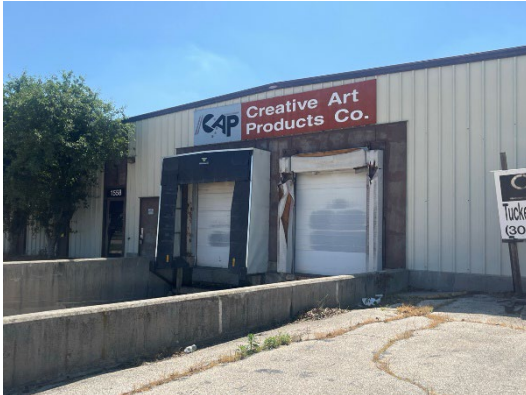
Deteriorated pavement, deteriorated loading dock.
