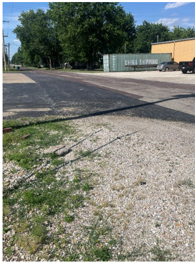
Deteriorated street pavement.
