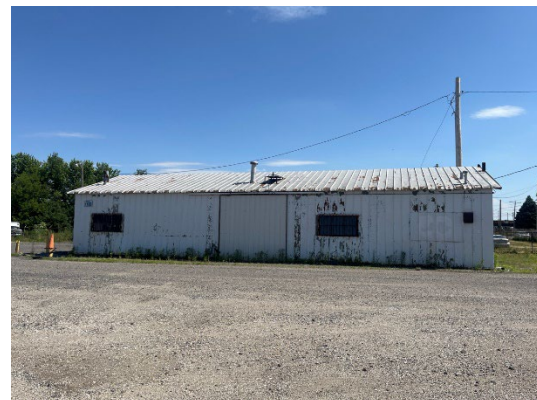
Boarded windows, aging metal roofing, lack of exterior maintenance
